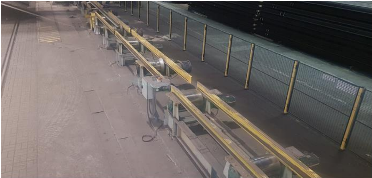
Figure 1 : Rail finishing area – line number 385
