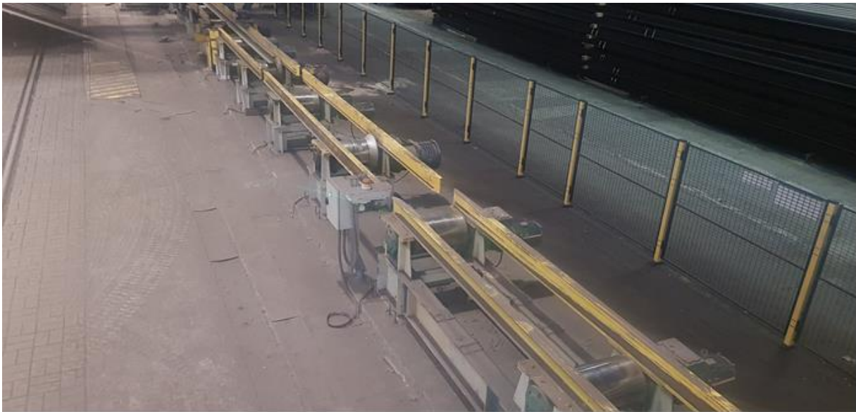
Figure 1 : Rail finishing area – line number 385
